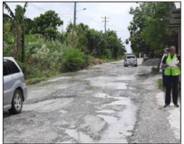
B: Waterlogged road near CH. 2900'
