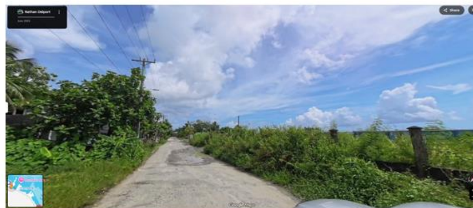
D: Pot holed road and overgrowth borders at Anaganan 1 km from Pou Bay Bridge.
