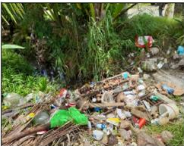
E: Culvert at Ch. 1428 filled with solid waste
