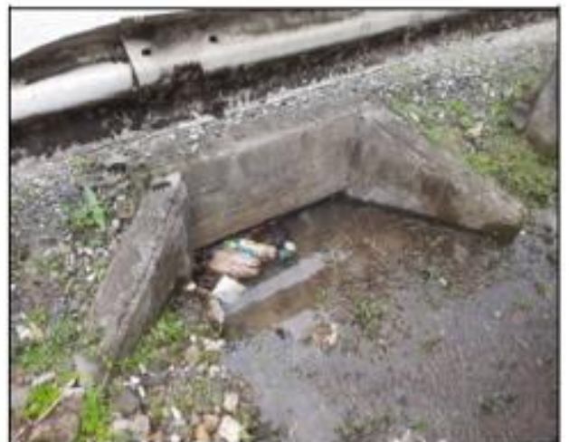
F: Choked culvert at CH. 4303
