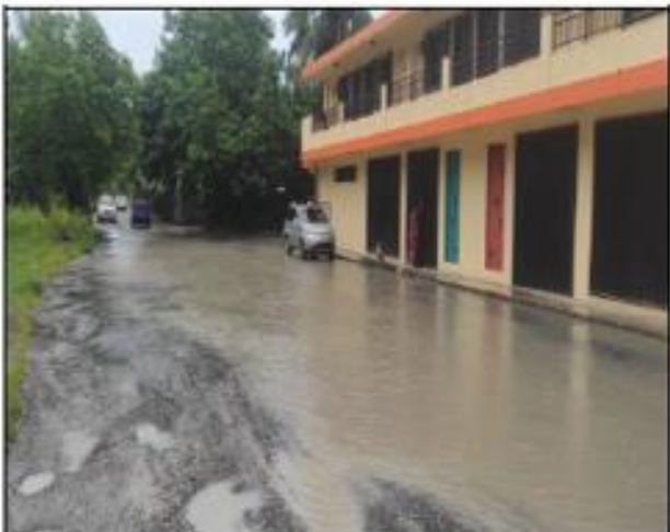
C: Waterlogged road near CH. 5570'
