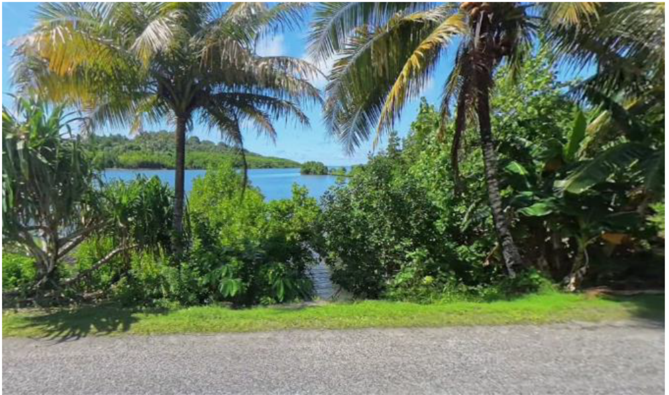
Figure 26: Vegetation at the culvert location on the eastern side of the Awak bridge - Ocean side (A)/ Mountain side (B)
