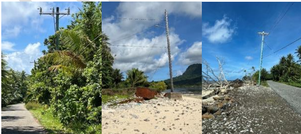
Figure 10 –Existing Power Pines, Kosrae State
